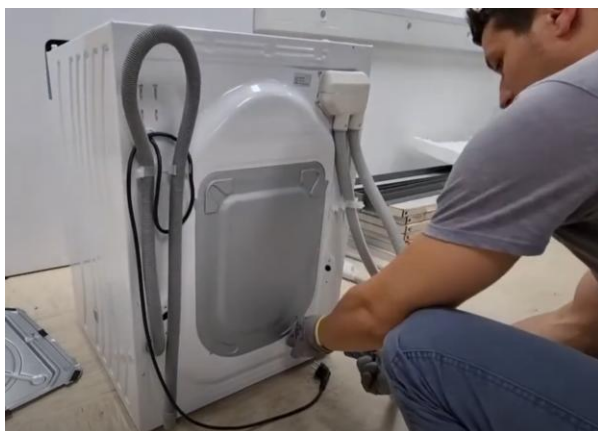
FIGURE 3: WASHING MACHINE MAINTENANCE
